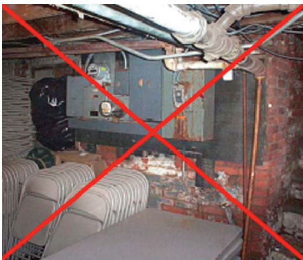
Electrical equipment rooms that are used for storage can create property and liability exposures.
