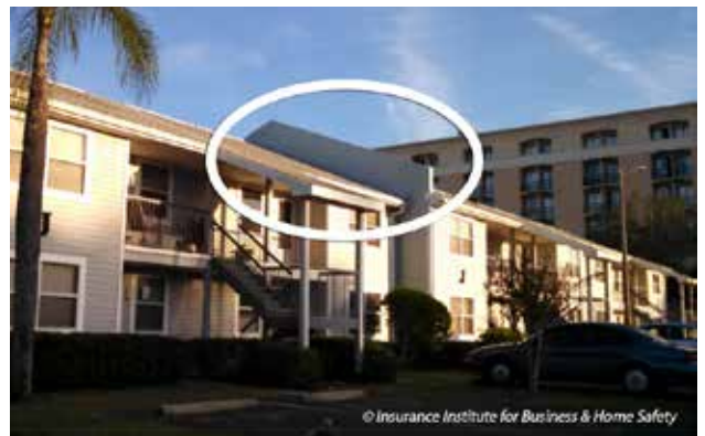
Fire wall separating two buildings—reducing the risk of a fire jumping from one roof to another
