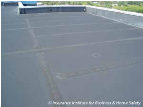
Single-ply EPDM membrane roof cover (mechanically attached).
