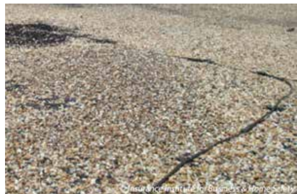
Built-up roof cover with gravel embedded in asphalt. (A lightning protection cable also is shown.)
