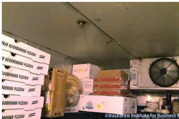
Sprinkler head located at the ceiling of this walk-in cooler.
