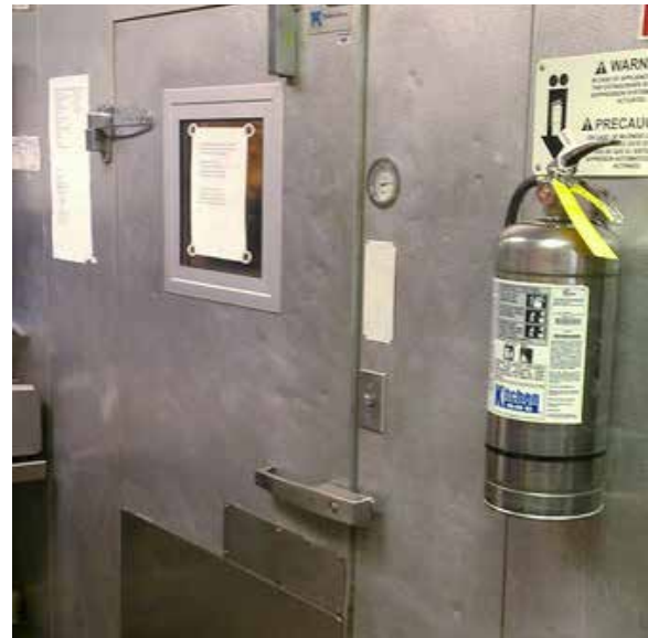
Typical walk-in cooler.
